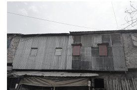
Various types two-storey of CI sheet (Tin) roof shades and facade windows in the settlement
