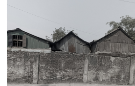
Poor facade condition observed from the outside of the settlement
